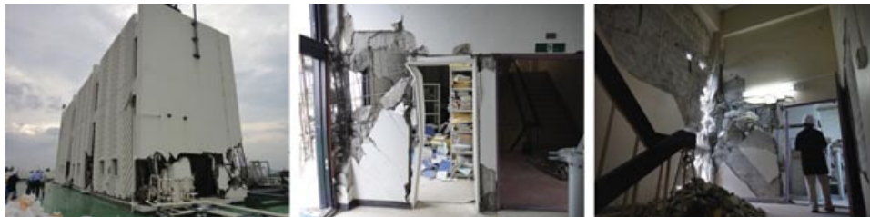
Figure 2. The building suffered significant structural damage due to the earthquake.
